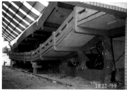
Photo 1 Strong-beam and weak-column failure of school building
